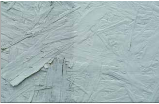
Figure 16–11. Absorption of water causes differential dimensional change of surface flakes to give an uneven surface (telegraphing).
